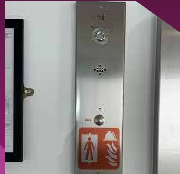
Figure 3 - Firefighters Lift facility accessible from the main entrance.
