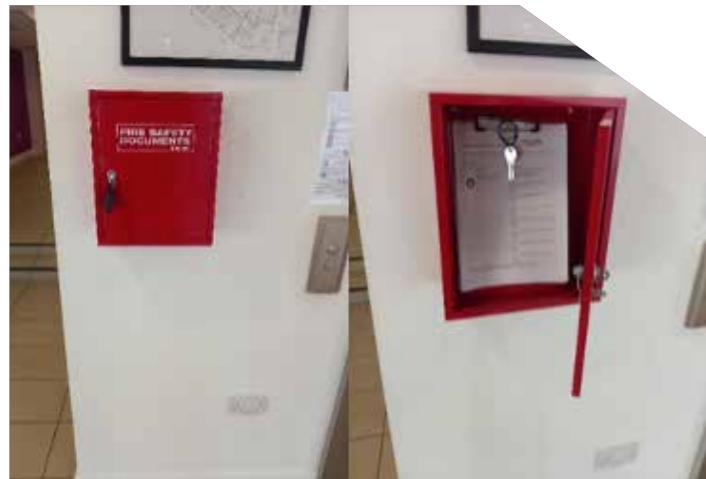
Figure 8 - Premises Information Box installed at Crocodile Court Y Block
